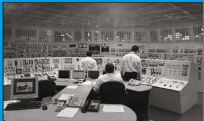
Conventional nuclear power plant control room
